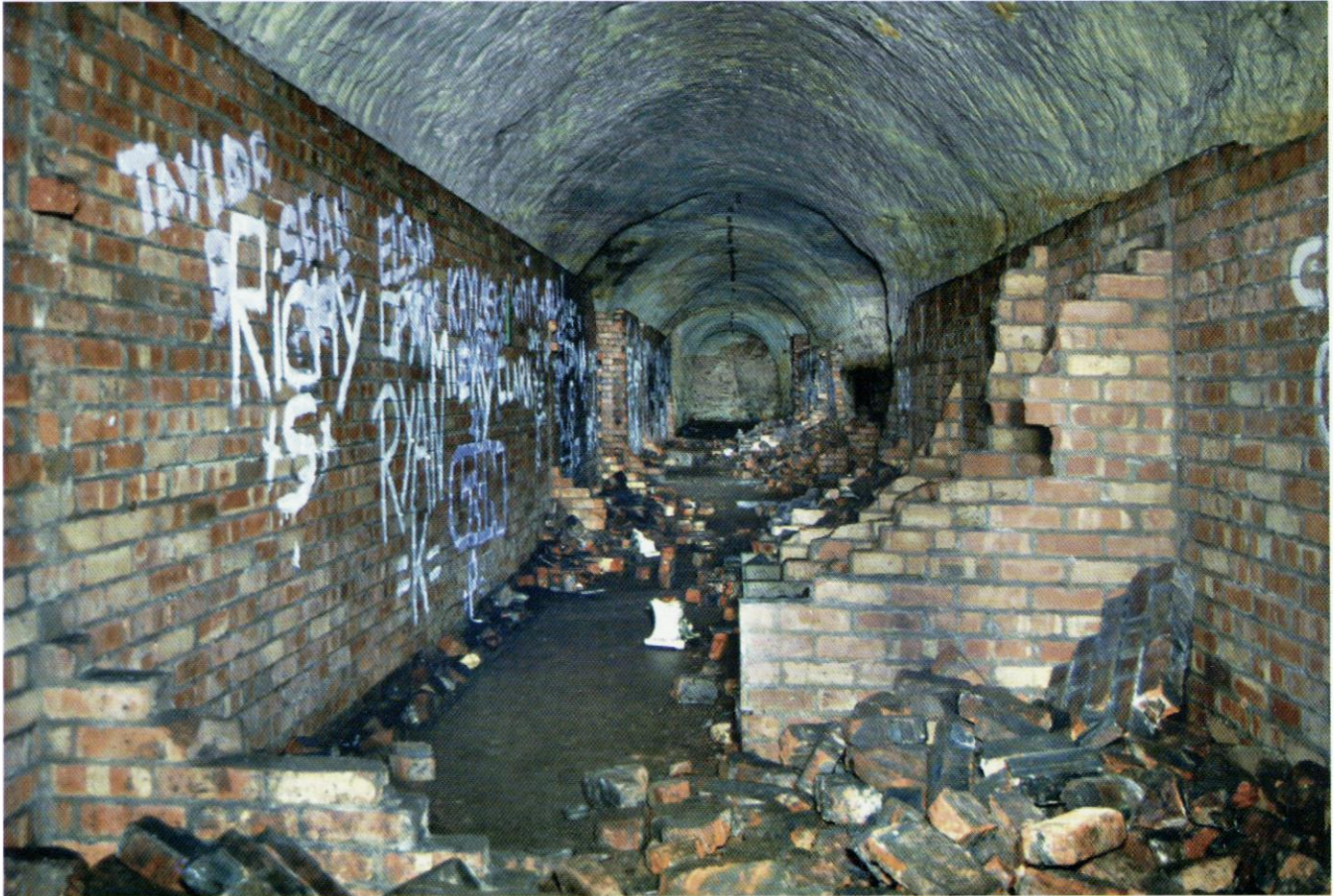
Bidston is one of two large civilian shelters under the sandstone hills of Bidston and Tranmere in the Wirral, across the Mersey from Liverpool. Photo Chris Rayner
